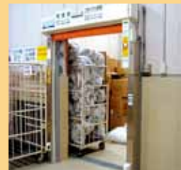
▲Installation example (Supermarket)
