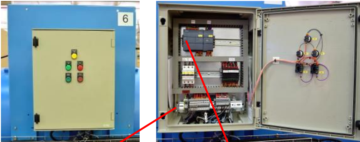
The Slave Control Panel
