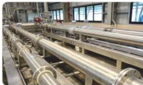
Piping system II (Maximum diameter is 500mm)
