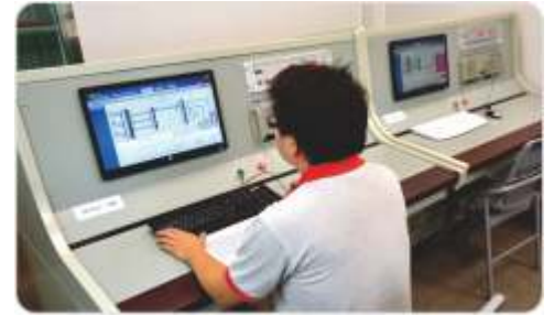
Control room & Graphical HMI
