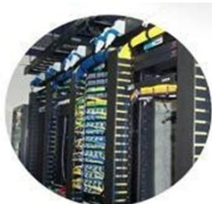
Optical fiber communication room
