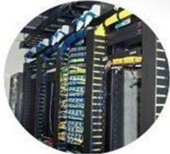
Optical fiber communication room
